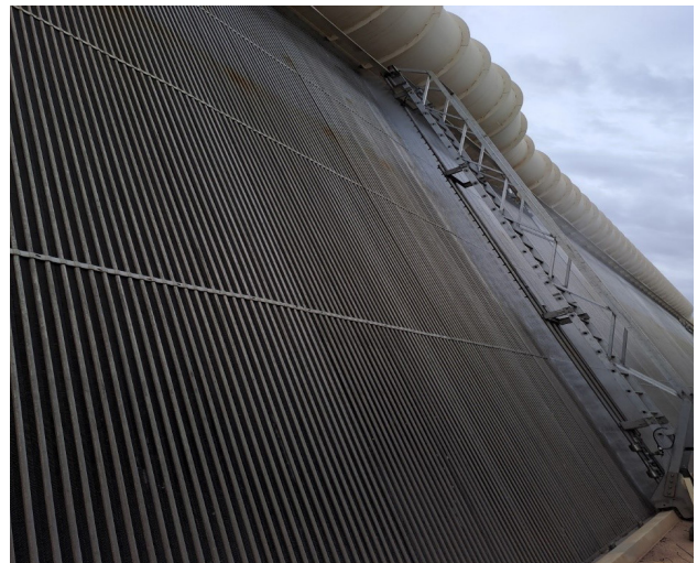
Figure 12. ACC Washing System
